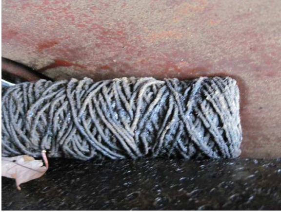
Failed unraveled Micron filter.
