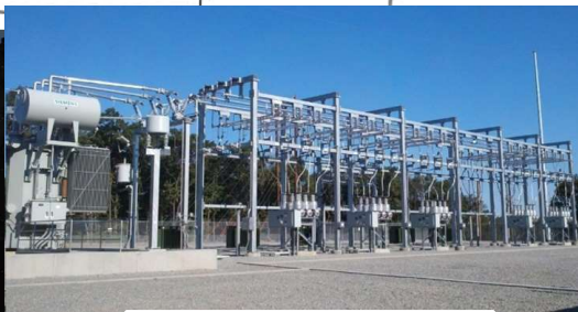
DLC 390 Transmission & Distribution Substations
