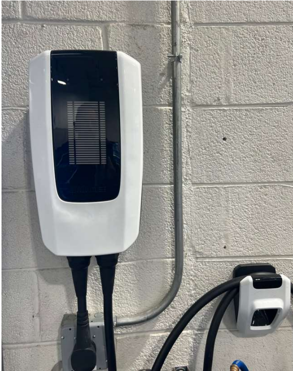
Residential EV charger – 11.5kW
